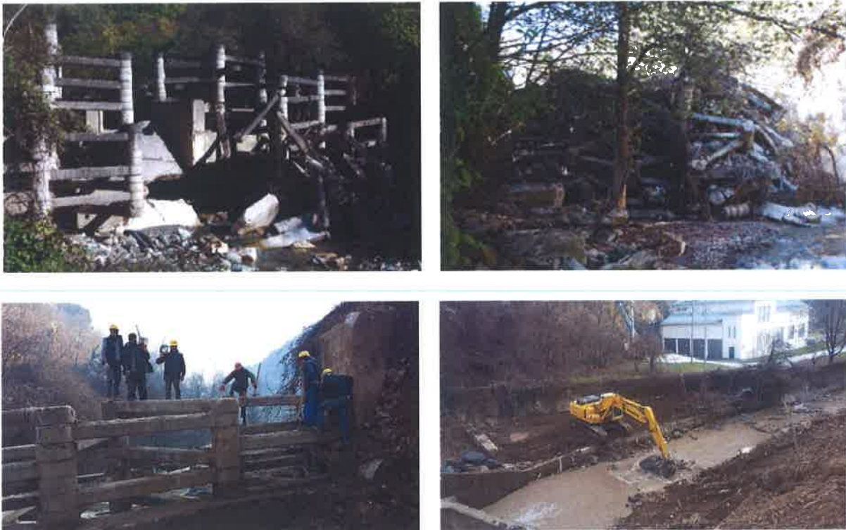
Fig. 3. Check-dams on the Pena River after the flash floods on 3 August 2015 and ongoing reconstruction
